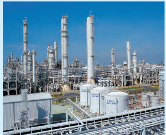
工廠排水配管 Petrochemical plant
